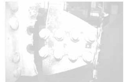
Figure 2-14. Tension Rupture. (From: Manual of Steel Construction, 9th Edition, Copyright © 2001, American Institute of Steel Construction, Inc.)
