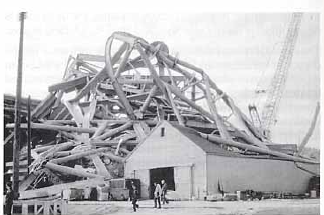
Figure 1.15 Stability and the strength of a structure—the collapse of a portion of the UW Husky stadium during construction (1987) due to a lack of adequate bracing to ensure stability. Photo by author.
