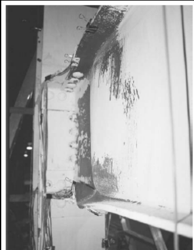
Figure 2-7. Web Local Buckling Limit State (SAC Project)
