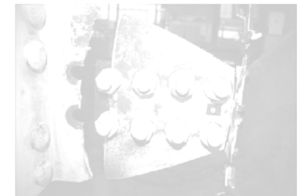
Figure 2-14. Tension Fracture Limit State (Photo by J.A. Swanson and R. Lyon, courtesy of Georgia Institute of Technology)
