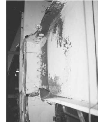
Figure 2-7. Web Local Buckling Limit State (SAC Project)
