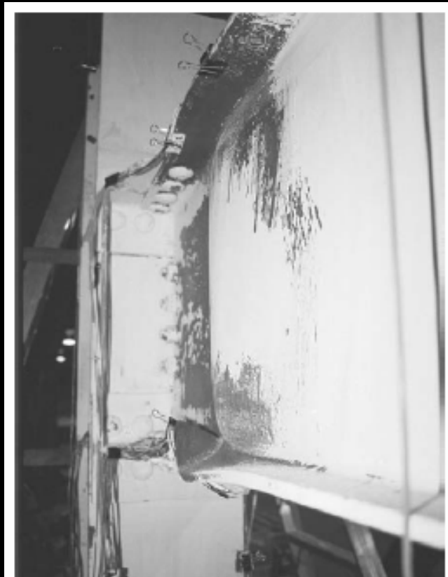
Figure 2-7. Web Local Buckling Limit State (SAC Project)
