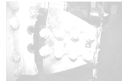
Figure 2-14. Tension Rupture Limit State (Photo by J.A. Swanson and R. Lyon, courtesy of Georgia Institute of Technology)
