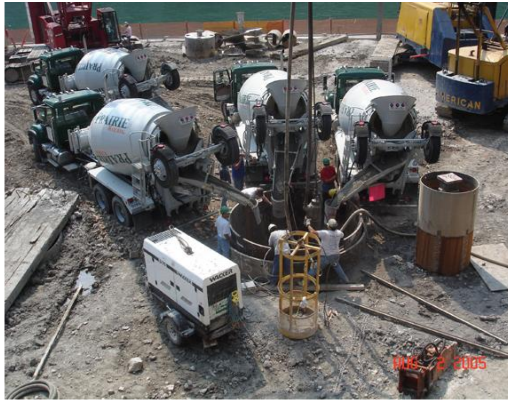
Three truckloads and 30 cubic yards of concrete discharged in 60 seconds into 10ft diameter Tower caisson
