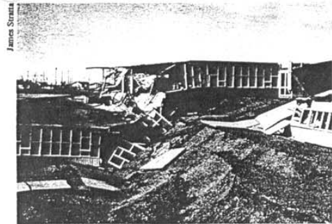
Figure 1.3: School straddling a landslide-induced rupture, Alaska
