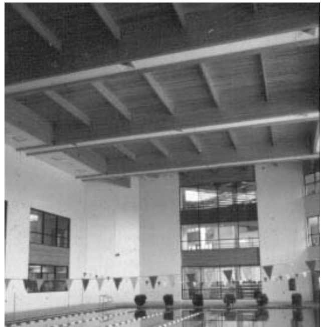
YMCA Pool, Brewton, AL; Architect—Dampier and Associates; Structural Engineer—Joseph and Spain; Contractor—Stuart Construction
