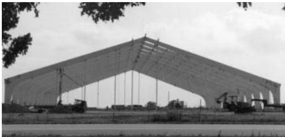
Animal Science Center, 172 ft. span arches, Univ. of Arkansas, Little Rock, AR; Architect--AMR Architect; Structural Engineer--Engineering Consultants, Inc.; Contractor--Harrison Davis Construction
