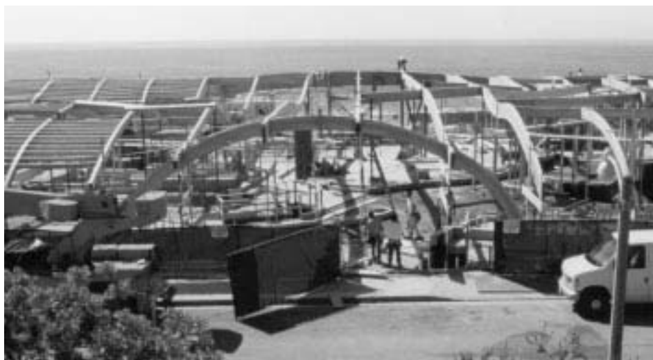
Newport Beach, CA, 30,000 sq. ft. residence; Architect--Brian Jeannete and Associates; Structural Engineer--Omnispan Corporation; Contractor--Buwalda Construction
