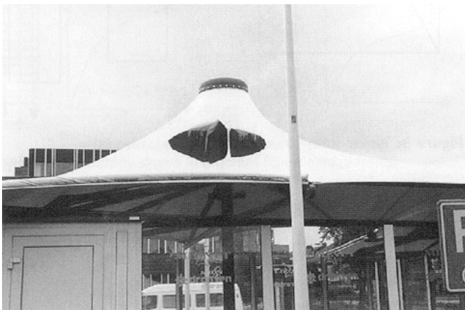
Fig. 2a PVC coated Polyester structure in the Netherlands After local fire a hole occurs in the membrane, but the fabric itself is not destroyed.
