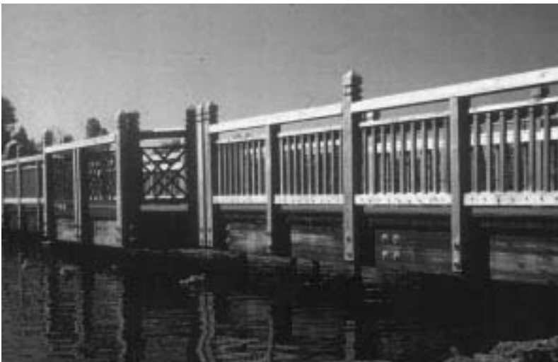
Bridge in Nature Park, Portland, OR, pressure treated with environmentally friendly copper naphthenate. Structural Engineer—Ceccacci Associates.
