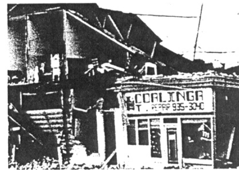
Figure 1.12: Damage to an older masonry building
