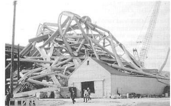
Figure 1.15 Stability and the strength of a structure—the collapse of a portion of the UW Husky stadium during construction (1987) due to a lack of adequate bracing to ensure stability. Photo by author.
