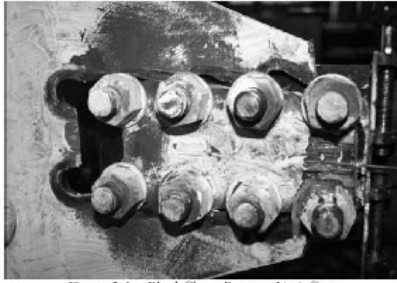
Figure 2-1. Block Shear Rupture Limit State (Photo by J.A. Swanson and R. Leon, courtesy of Georgia Institute of Technology)
