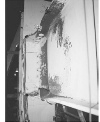
Figure 2-7. Web Local Buckling Limit State (SAC Project)
