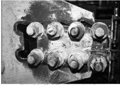
Figure 2-1. Block Shear Rupture Limit State (Photo by J.A. Swanson and R. Leon, courtesy of Georgia Institute of Technology)
