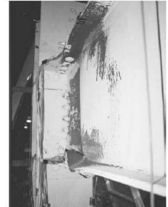
Figure 2-7. Web Local Buckling Limit State (SAC Project)
