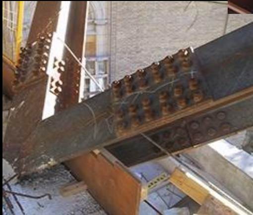
The Royal Ontario Museum Toronto, Canada Daniel Libeskind (AISC - Steel Structures of the Everyday)
