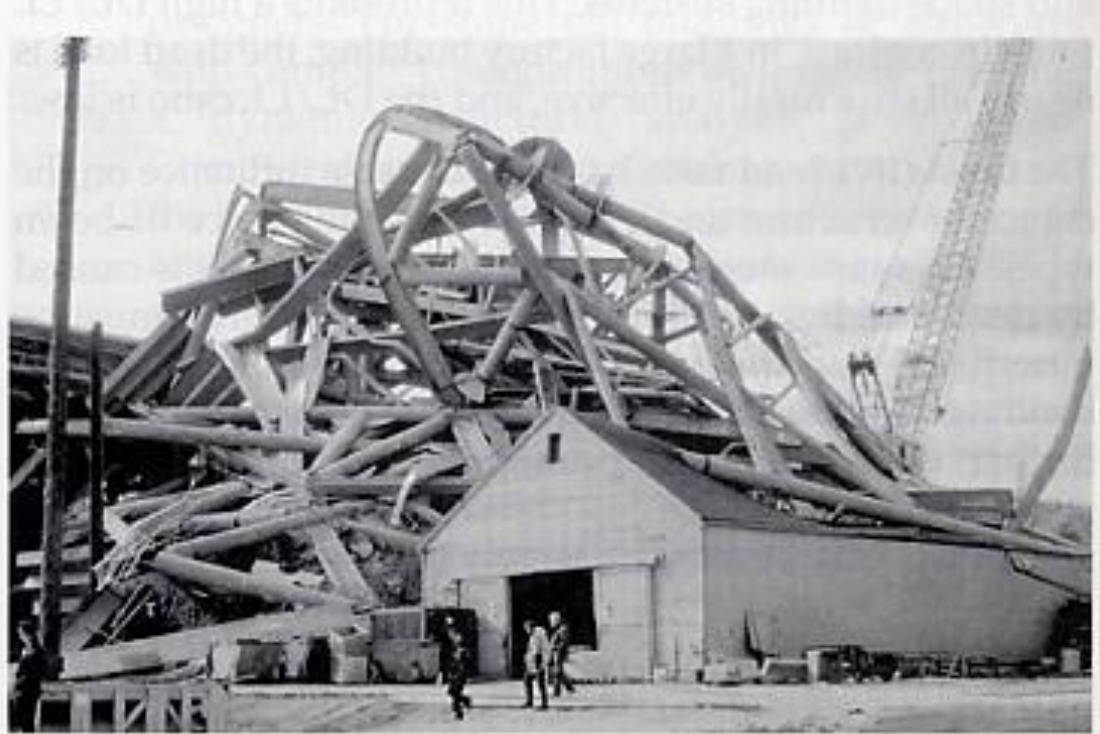
Figure 1.15 Stability and the strength of a structure—the collapse of a portion of the UW Husky stadium during construction (1987) due to a lack of adequate bracing to ensure stability. Photo by author.
